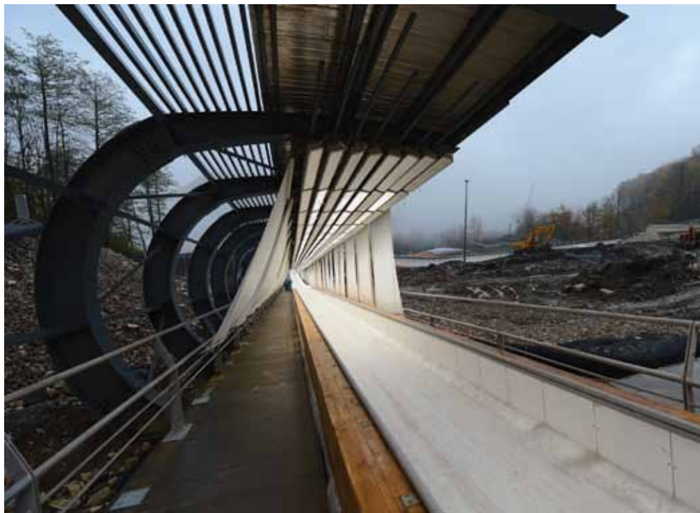
Above photo: A view of the construction of the Sliding Centre Sanki venue for Bobsleigh and Skeleton at the 2014 Winter Olympics on November 7, 2012 in Sochi, Russia.
