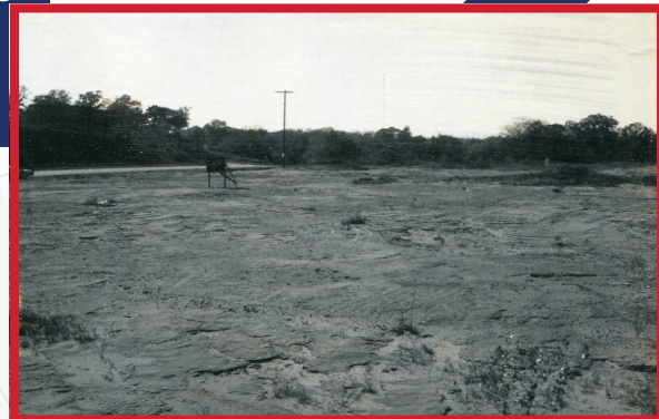
An early look at construction on the USA Softball (ASA) National Office in Oklahoma City.
